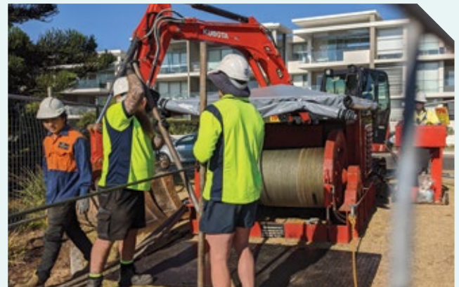
Laying cable (Source: Queensland Capacity Network Pty Ltd, trading as QCN Fibre)
