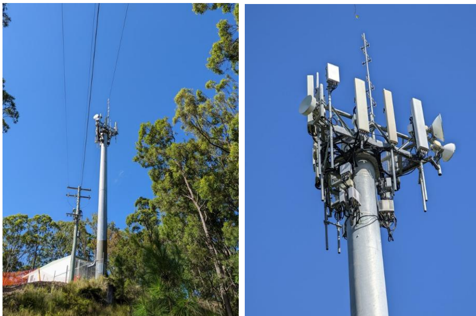
Figure 3: Existing telecommunications facility hosting Telstra equipment. (Source: RFNSA, 2025)
